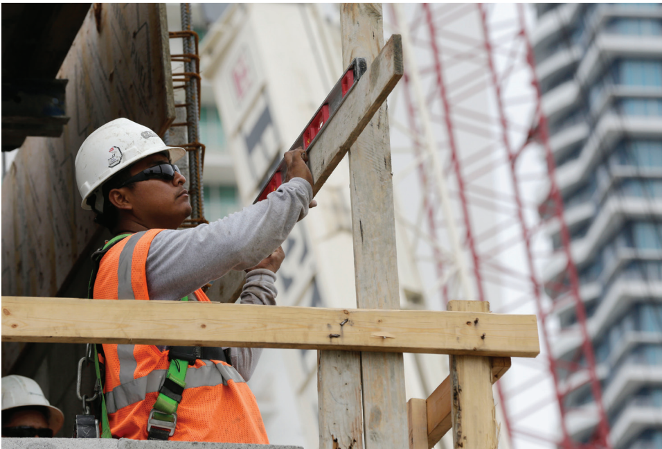
A construction worker on the site of the SoMa at Brickell apartment building in downtown Miami (AP Photo/Lynne Sladky)
